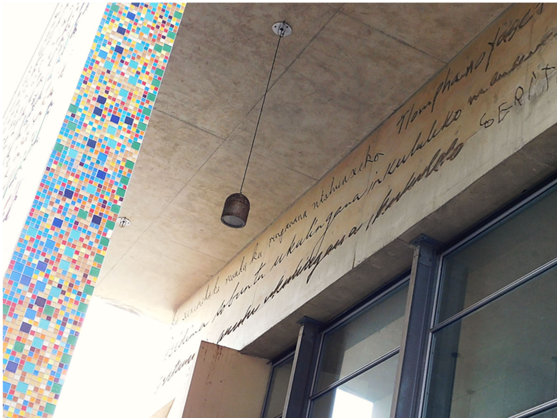
Figure15: View of one of the concrete beams at the entrance of the foyer with judges handwriting. Source: Author
