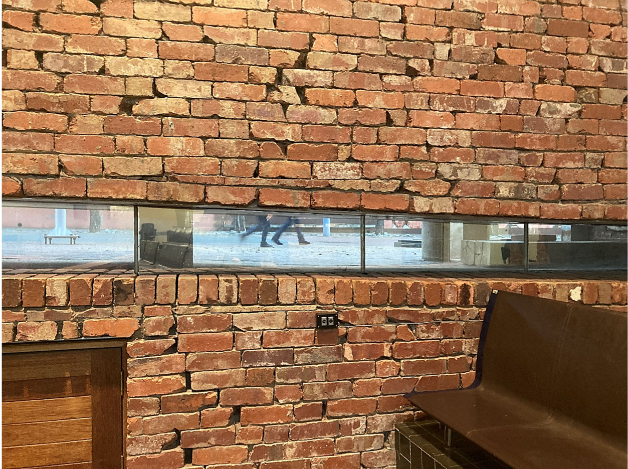
Figure 23: Image of narrow window along the brick wall of the court chamber
