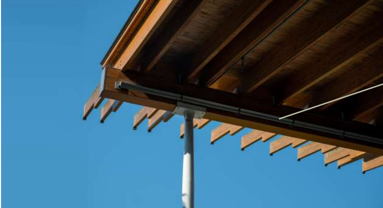
Added lighting with bird spikes
