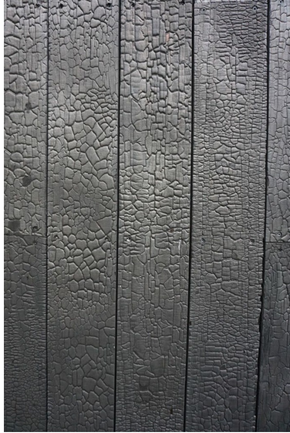
Figure 12: Burnt Timber Cladding
