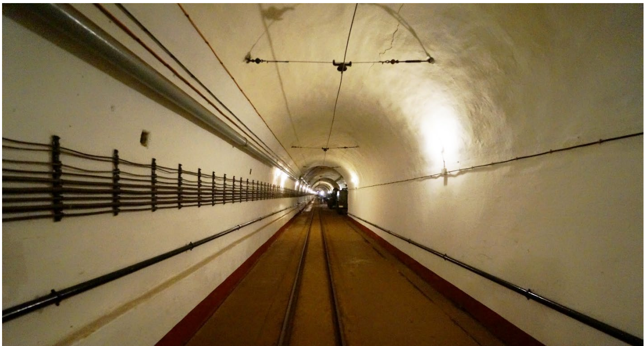
Fig. 9. Paul Painleve & C.O.R.F., the lifblood of the fort, telephone and electrical lines run the length of the tunnel, Ouvrage Hackenberg , Vekring, France, 1929-1932.
