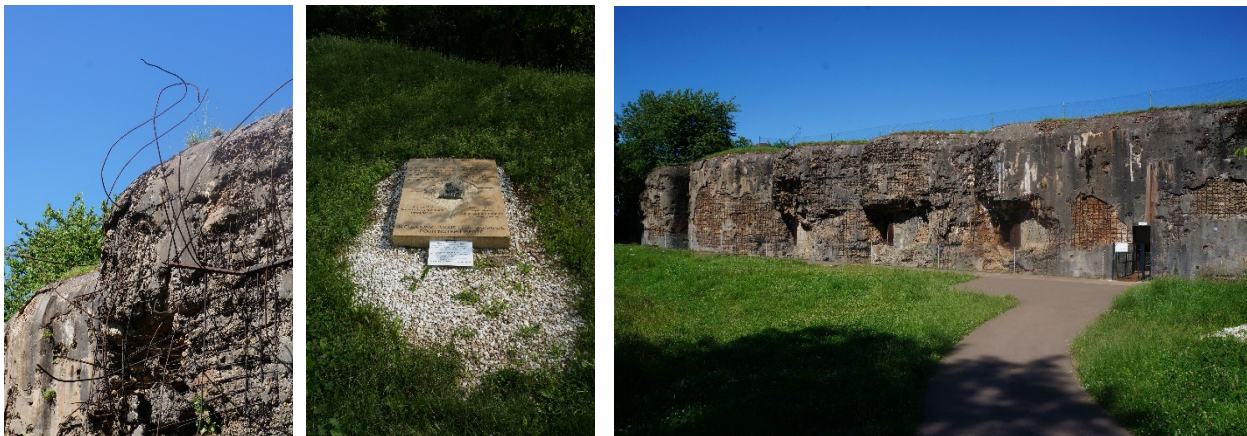
Fig. 12-14. Paul Painleve & C.O.R.F., views of Block 8's façade and adjacent American memorial with steel reinforcement exposed from the Allied assault, Ouvrage Hackenberg, Vekring, France, 1929-1932.
