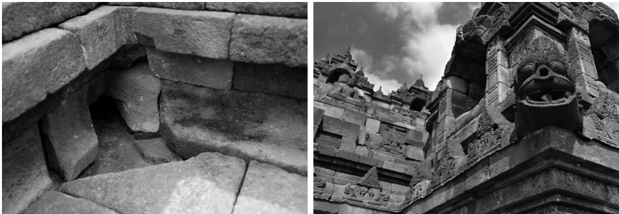
Figs. 13-14. Views of subtle rainwater management system, Borobudur, Yogyakarta, Java, Indonesia, 8 th -9 th centuries CE.
