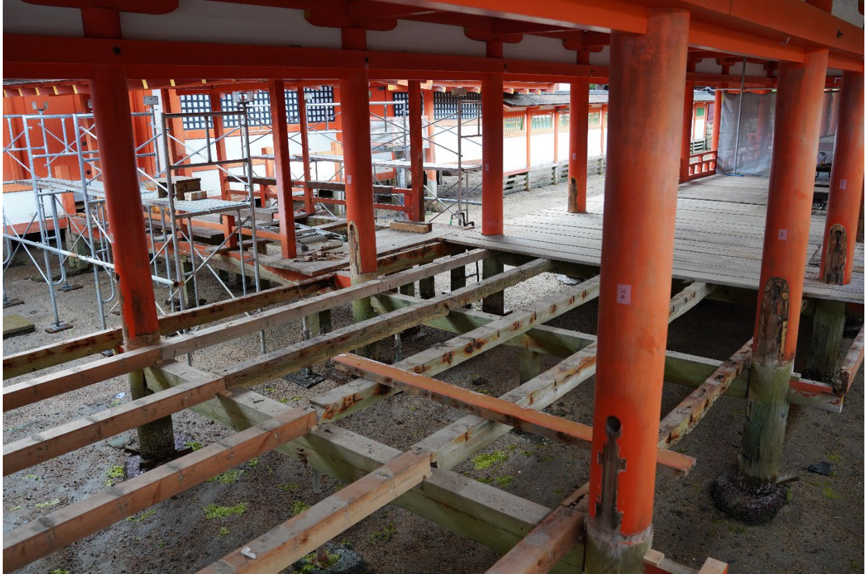
Fig. 31. Floorboards and the underlying structure are completely removed and replaced, Itsukushima Shrine, Hiroshima, Japan, 1168.
