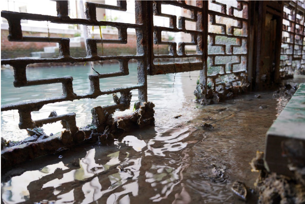
Fig. 22. View of the metal gates meeting directly with the water, Querini Stampalia, Venice, Italy, 1963.
