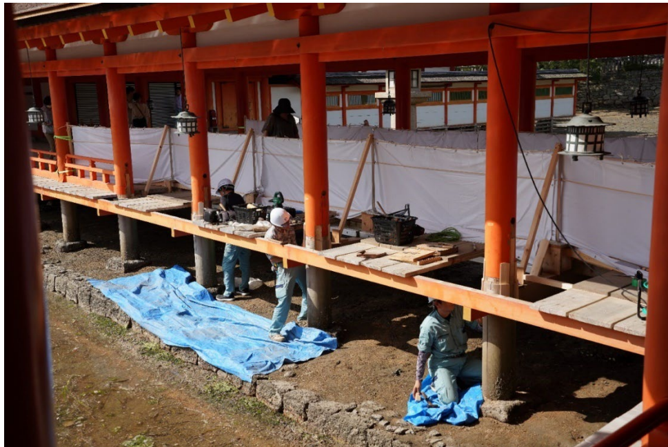
Fig. 34. Craftsman work by hand, during low tide, to splice brand new lower sections of pillars to existing upper sections, Itsukushima Shrine, Hiroshima, Japan, 1168.
