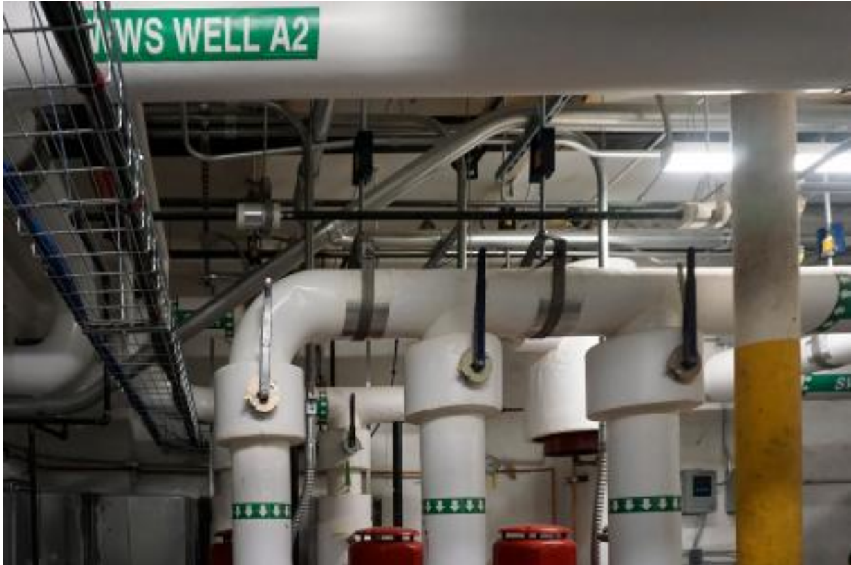
Fig. 17, Geothermal well, Colorado State Capitol Building, Denver, CO, 1894. Source: https://capitol.colorado.gov/projects/geothermal .
