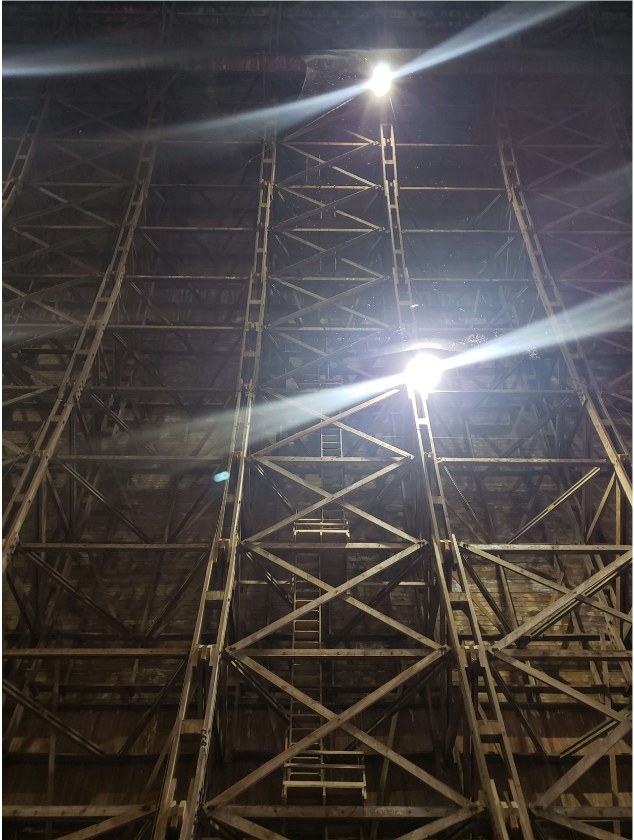
Fig. 7. Ladder as it climbs up the edge of the arched truss system, Tillamook, OR, 2021.
