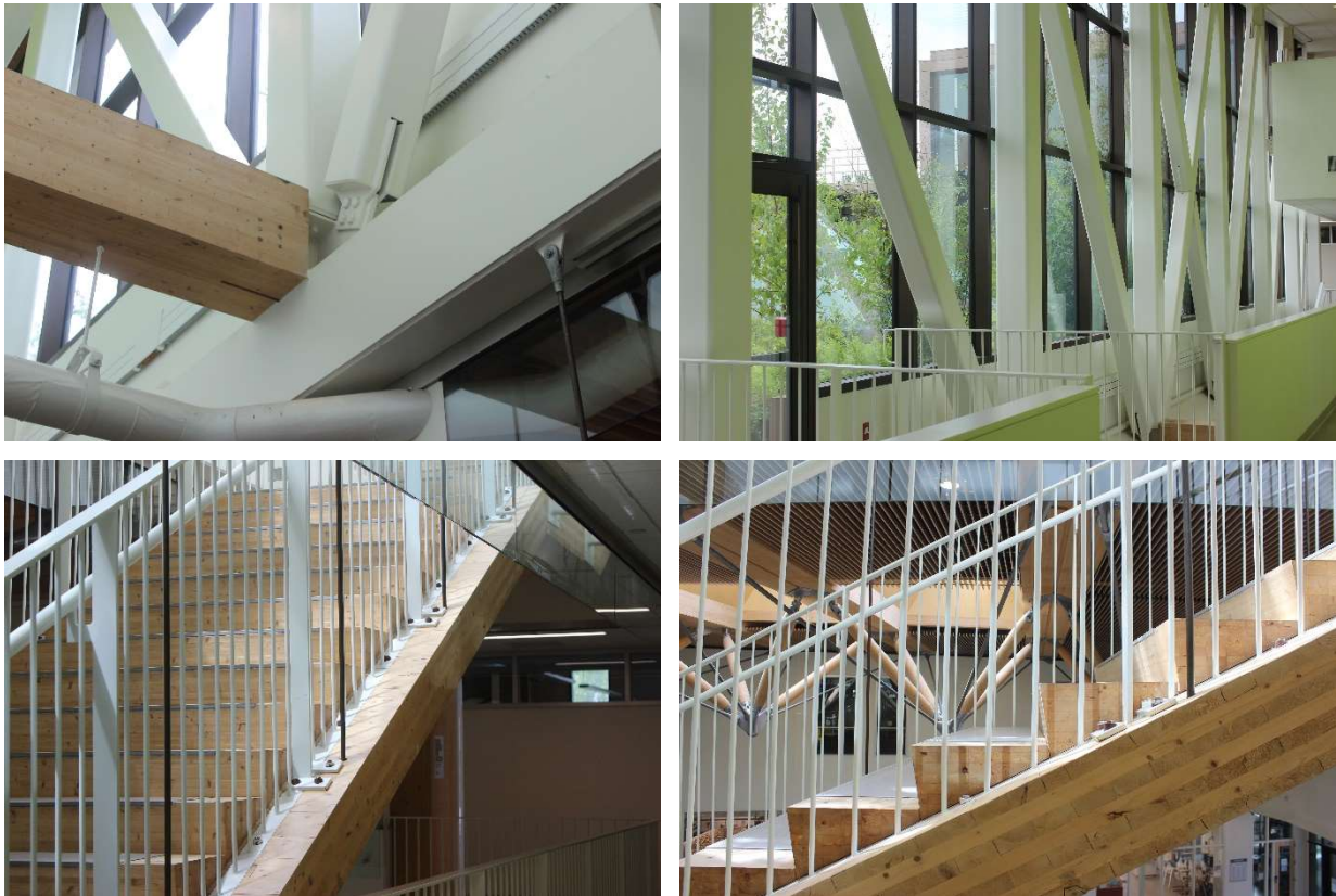
Fig. 8-9. Leers Weinzapfel Associates, views of the large steel truss that supports the north side of the zipper truss, John W. Olver Design Building, Amherst, MA, 2021.
