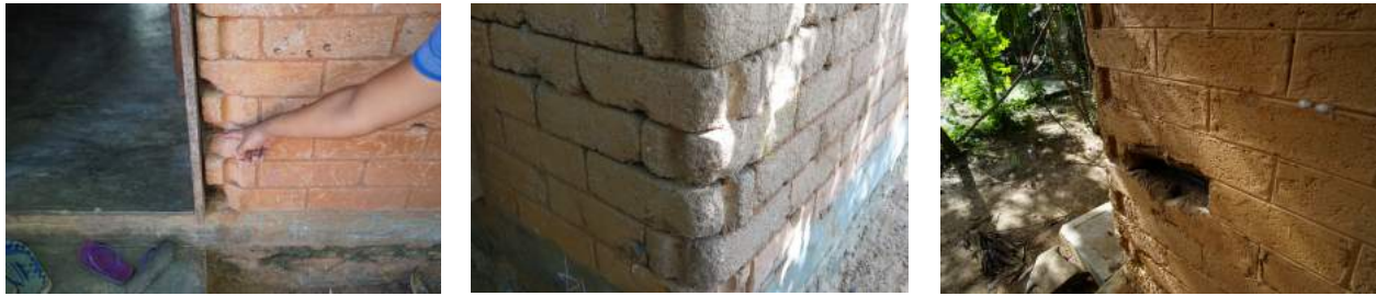
Fig. 23. Shigeru Ban, eroding and damaged earth blocks, Post-Tsunami Housing, Kirinda, Sri Lanka, 2007.
