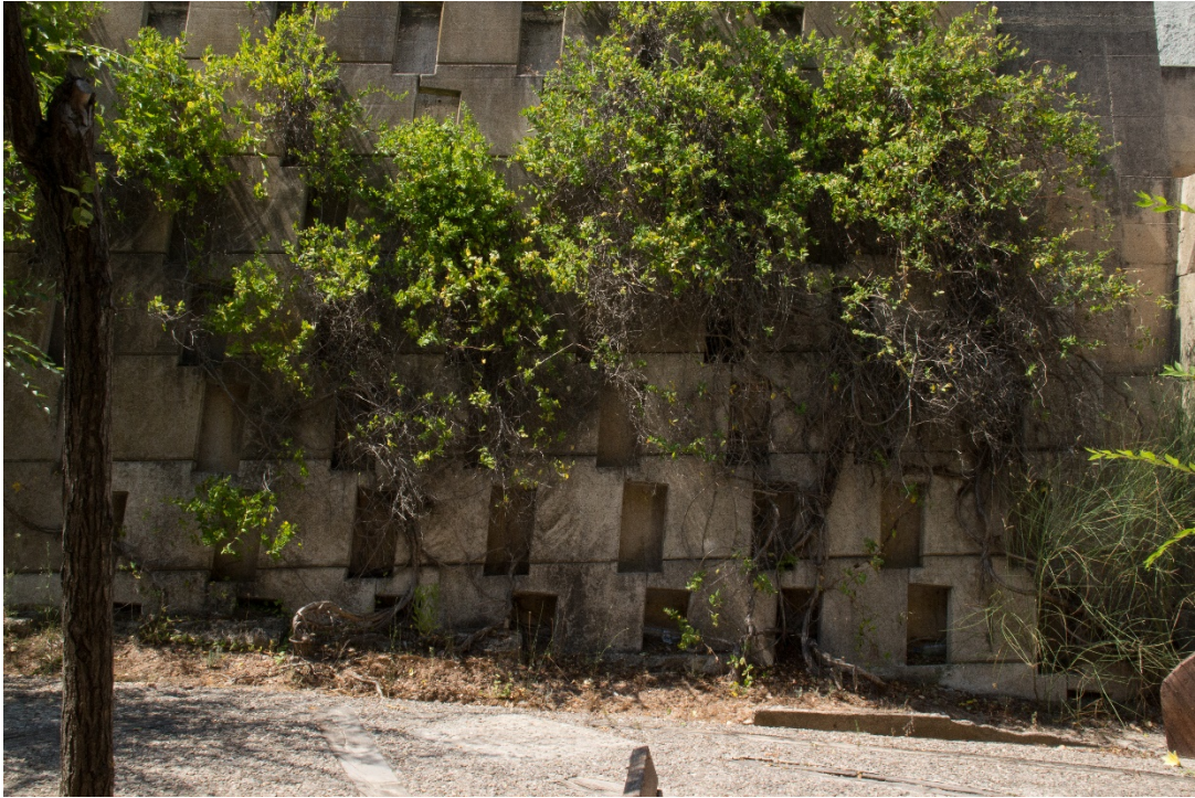
Fig. 30 - Vegetation on concrete
