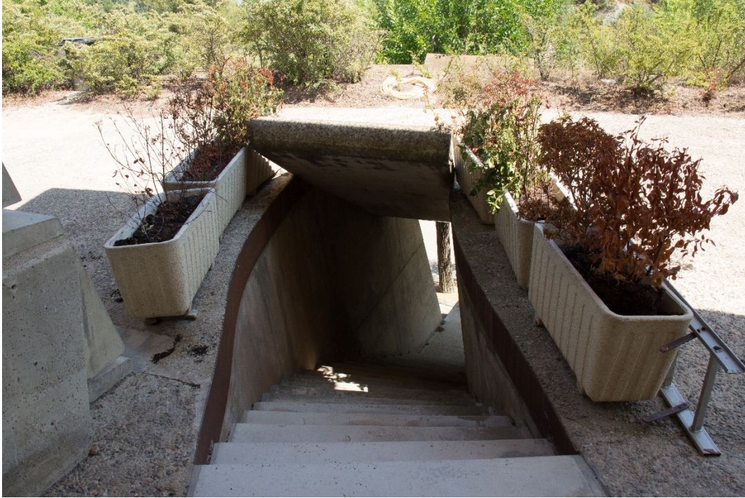
Fig. 21 - Protruding stairway opening
