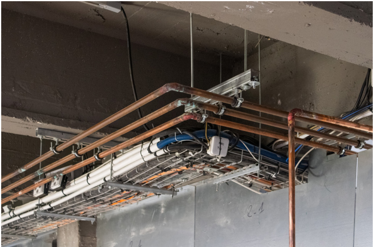
Fig. 10 Lacaton & Vassal, Electric Conduits with Piping installed by artist Mountaincutters , Palais de Tokyo, Paris, France, 2002. Photograph by author.
