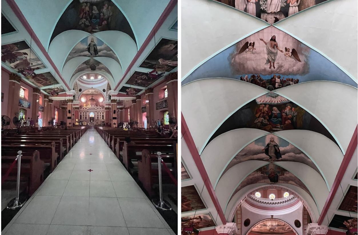
Fig.4. Binondo Church interior & ceiling detail | Manila, Philippines, Domingo de la Cruz González, 2023
